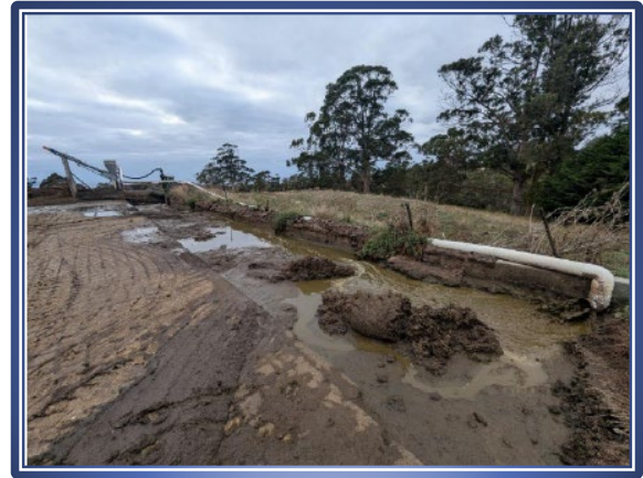
Figure 2-5 - Sump and trafficable solids trap
