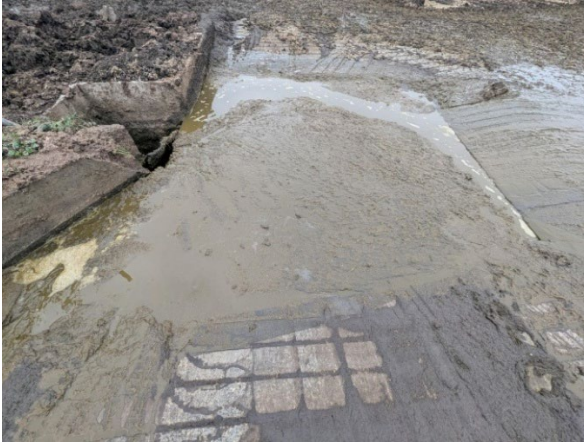
Figure 17. Drain collecting dairy and yard washdown, discharging to the TST and sump.
