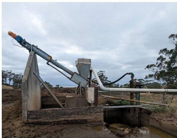
Figure 21. Sump on the eastern end of the TST with a screw press.
