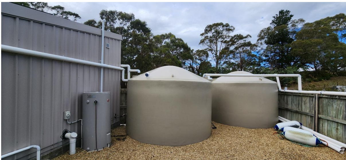
Current 2 x 14 000 litre water tanks
